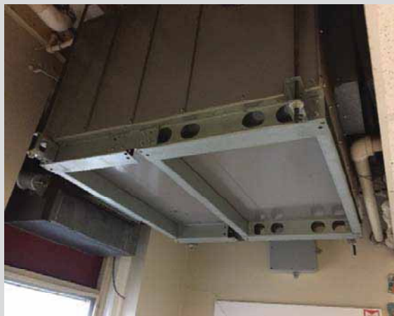
Existing Kitchen Make-up air unit
