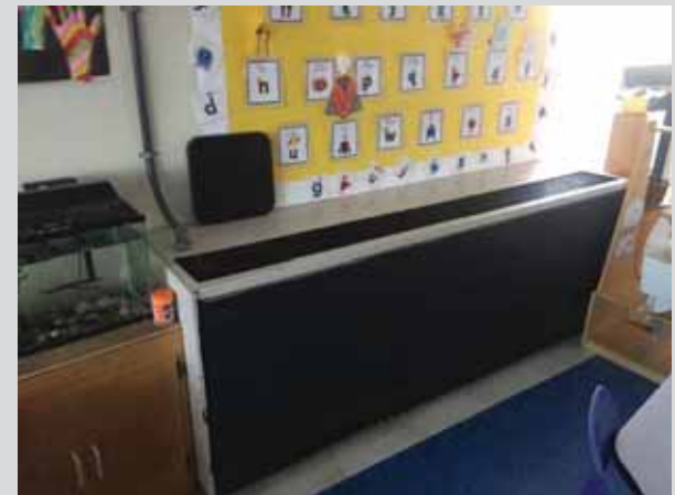
Typical Classroom Unit Ventilator
