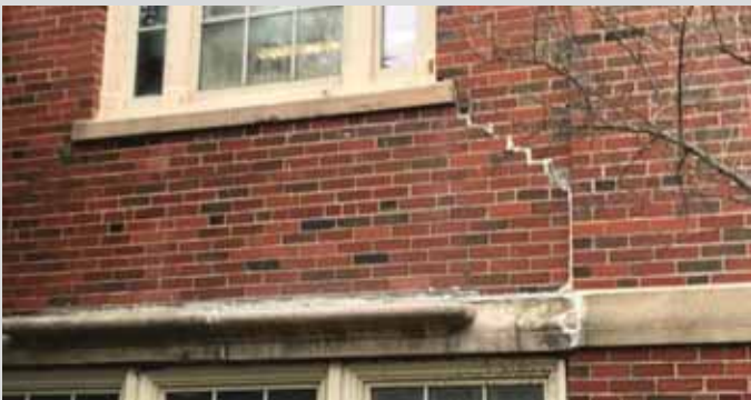
Brick and cast stone conditions
