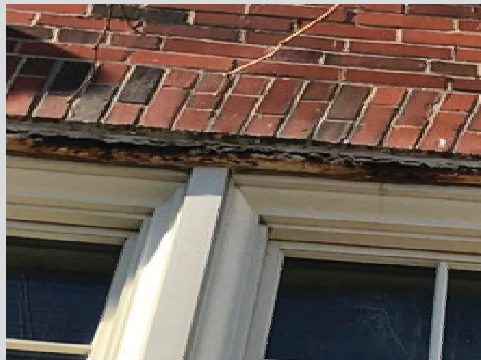
Rusted lintel conditions
