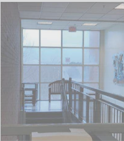
Failing Curtain Wall
