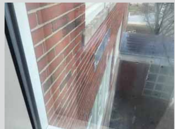
Typical intake for Classroom Unit Ventilator
