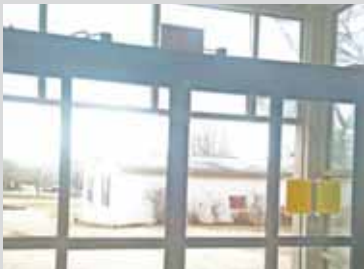
2. Magnetic locks and door position switches on the interior of the door.
