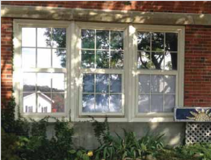
Majority of window seals have failed
