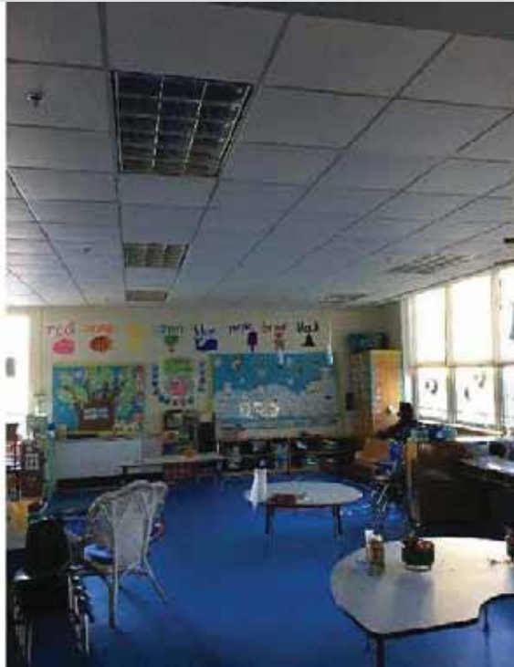
1997 Wing Classroom Lighting: 2'x4' Parabolic Fluorescent Fixtures: Fair Condition
