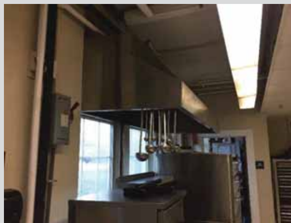
Existing Kitchen Hood • No Fire Suppression • Undersized, No Grease Trap
