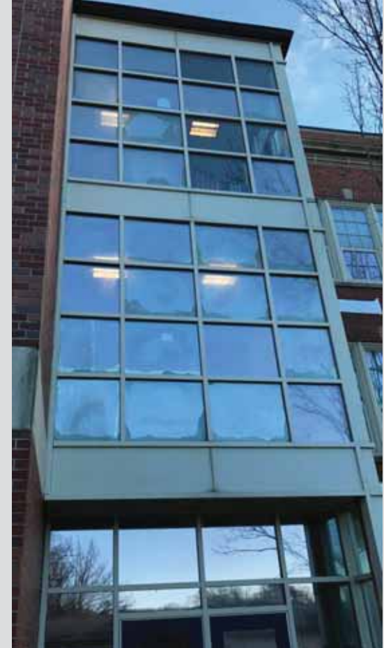
Curtainwall seals have failed
