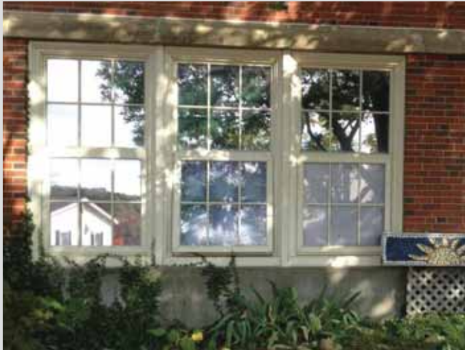
Majority of window seals have failed
