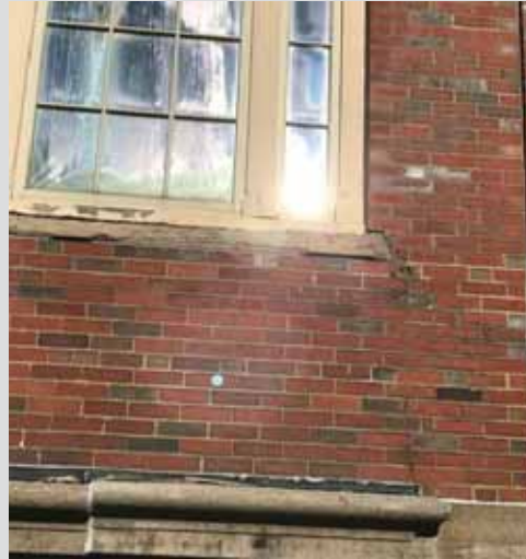
Deteriorated sill conditions
