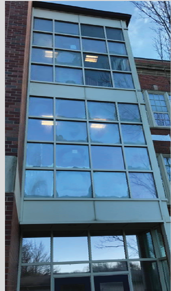
Curtainwall seals have failed
