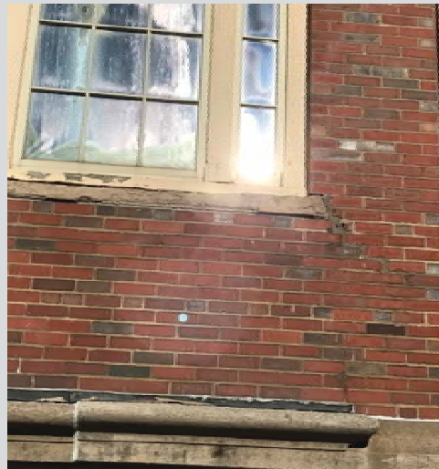
Deteriorated sill conditions
