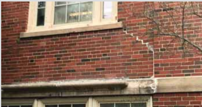
Brick and cast stone conditions
