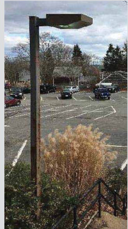
Pole Light Fixture: Poor Condition
