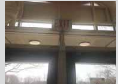
4. Request to exit and door position switches on the interior of the door.
